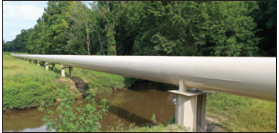
Above Ground Pipeline Crossing Cow Bayou
